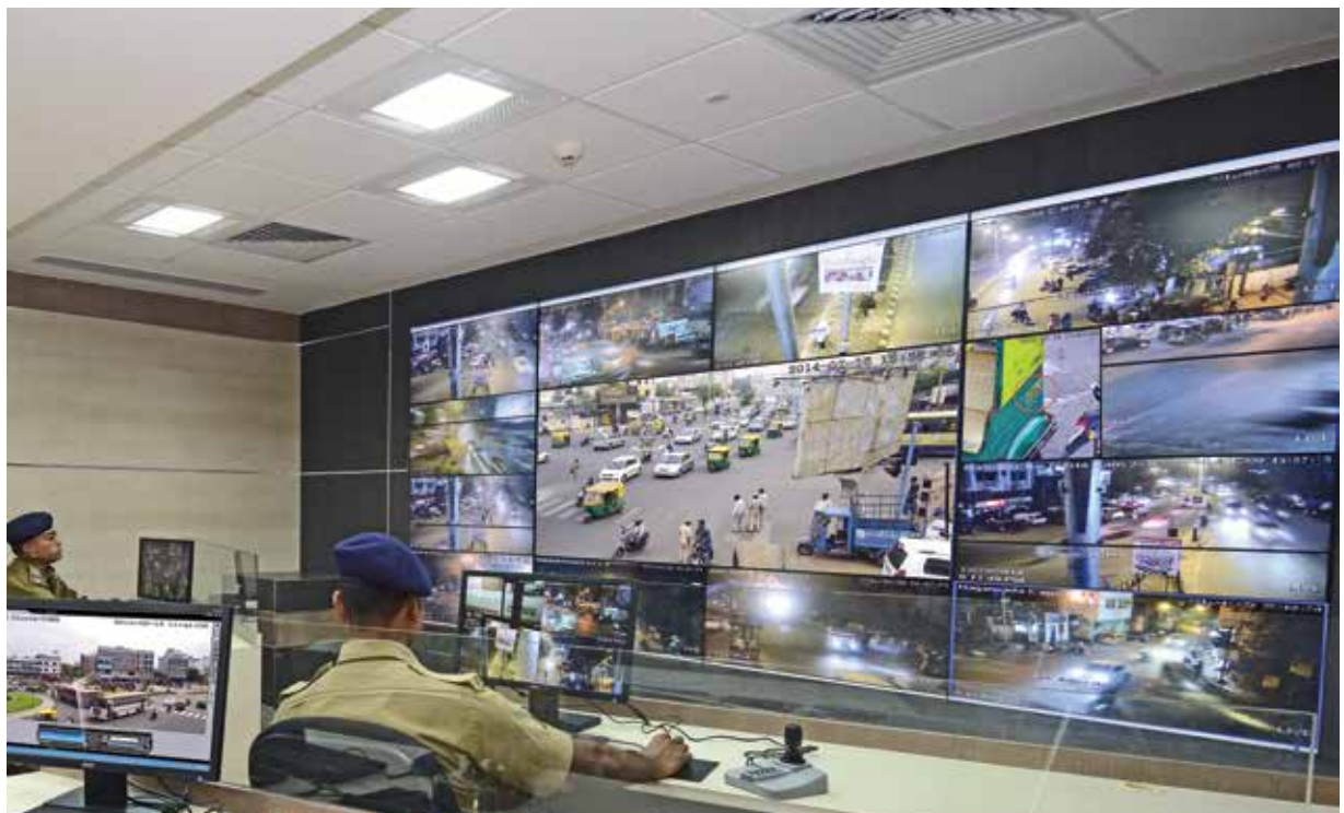
Gujarat CCTV project- L&T's prowess as a Master Systems Integrator (MSI), three key cities in Gujarat are now under 24/7 surveillance which eases traffic management and enhances vigilance. Putting together this state-of-the-art CCTV project consists of fixing a third eye at 288 locations.
