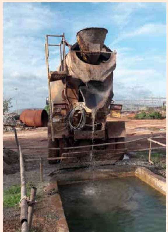
Waste Water Collection Tank
