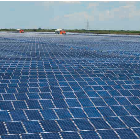
60 MWp Solar Tracker Plant at Tiruchuli, Tamil Nadu
